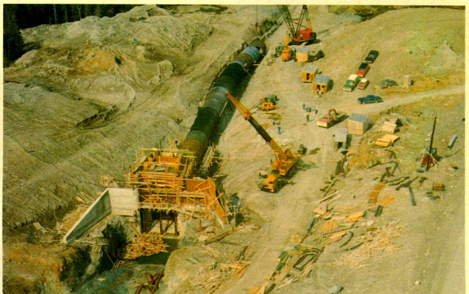
Intake and penstock construction for the hydro-electric generating plant at Hinds Lake with a capacity of 75 megawatts, scheduled to commence production in November of 1980.
