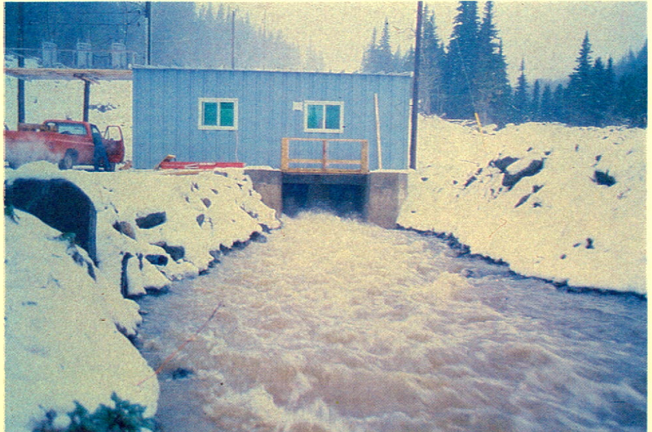
Mini-hydro plant at Roddickton in Northern Newfoundland went into operation in December, 1980. The plant was built under an agreement with the Government of Canada.
