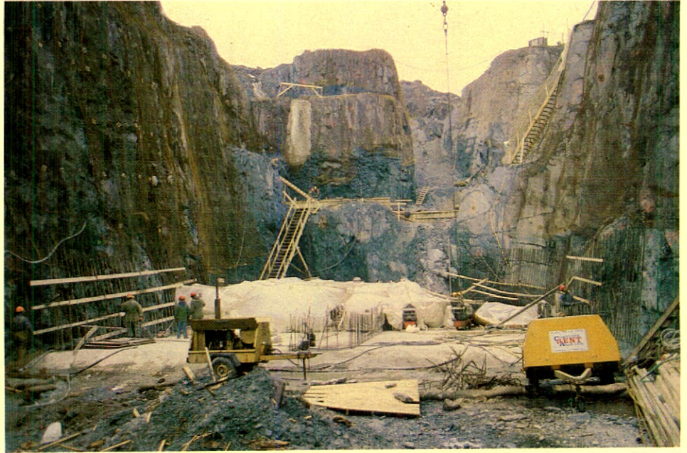
Excavation for the powerhouse at the Upper Salmon hydro-electric project. The plant will cost $155 million and displace 830,000 barrels of oil annually.
