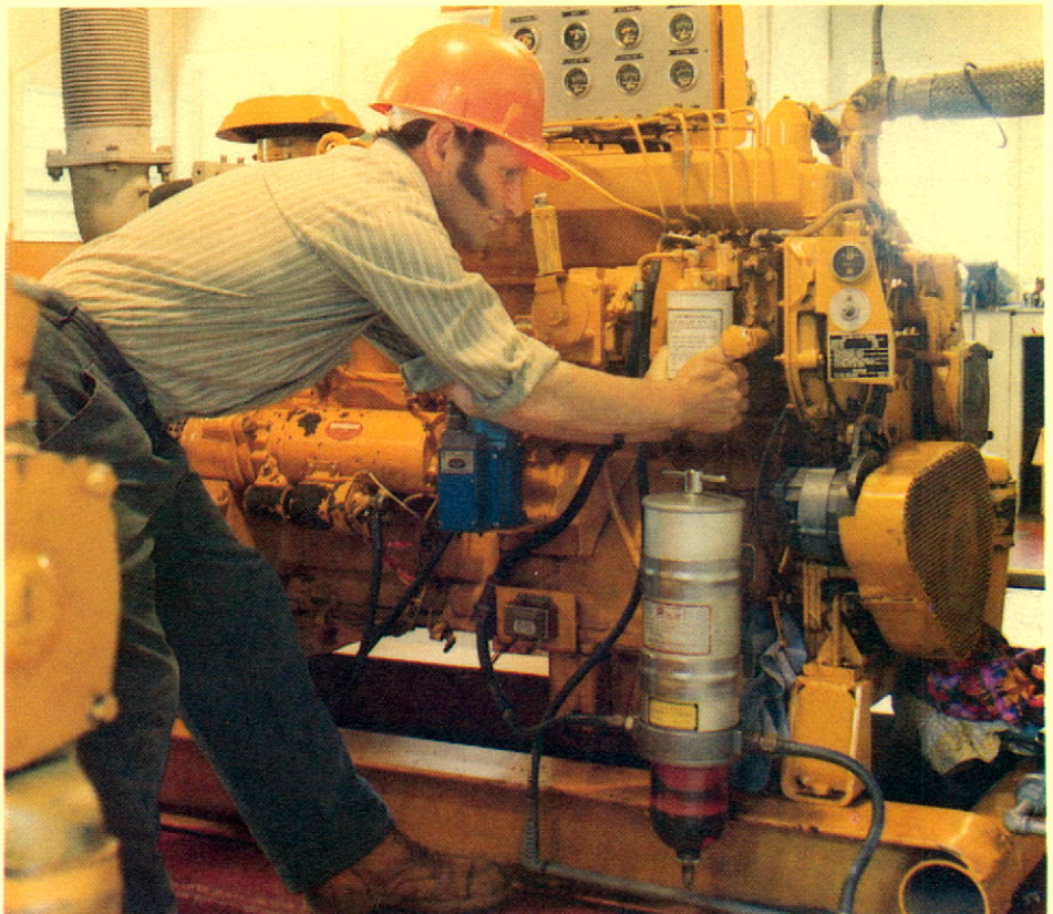
Diesel plant operator performing regular maintenance work on one of the 44 diesel generator plants operated by the Power Distribution District.
