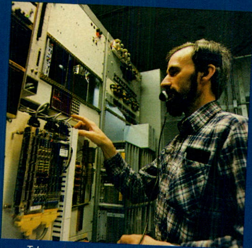
Telecontrol Supervisory Technologist at Hinds Lake Hydro-electric Generating Plant
