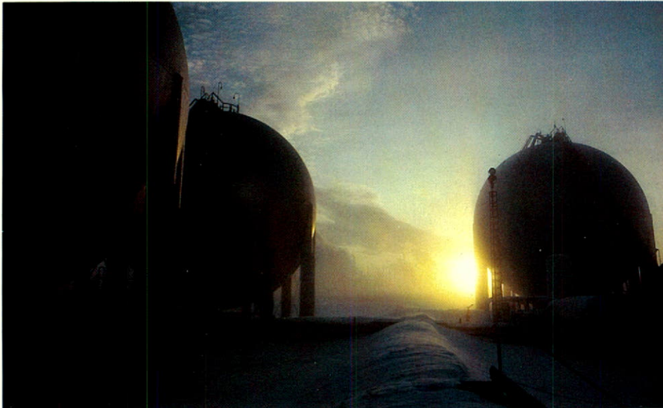
Company Horton-spheres in Edmonton store NGL. Dome's extensive storage facilities for liquids, both underground and above-ground, help assure delivery to customers at times of peak demand.
