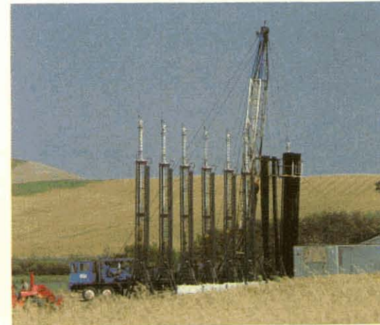
Specialized pumping system is used for enhanced heavy oil recovery at Morgan, Alberta, 115 miles east of Edmonton, near the Saskatchewan border.
