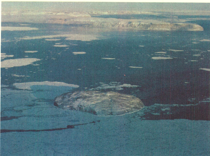
Above left: Tarsiut drilling island was built in 75 feet of water with sand-filled caissons. Its steep 1:5 slope minimized need for dredging and made possible faster completion.
