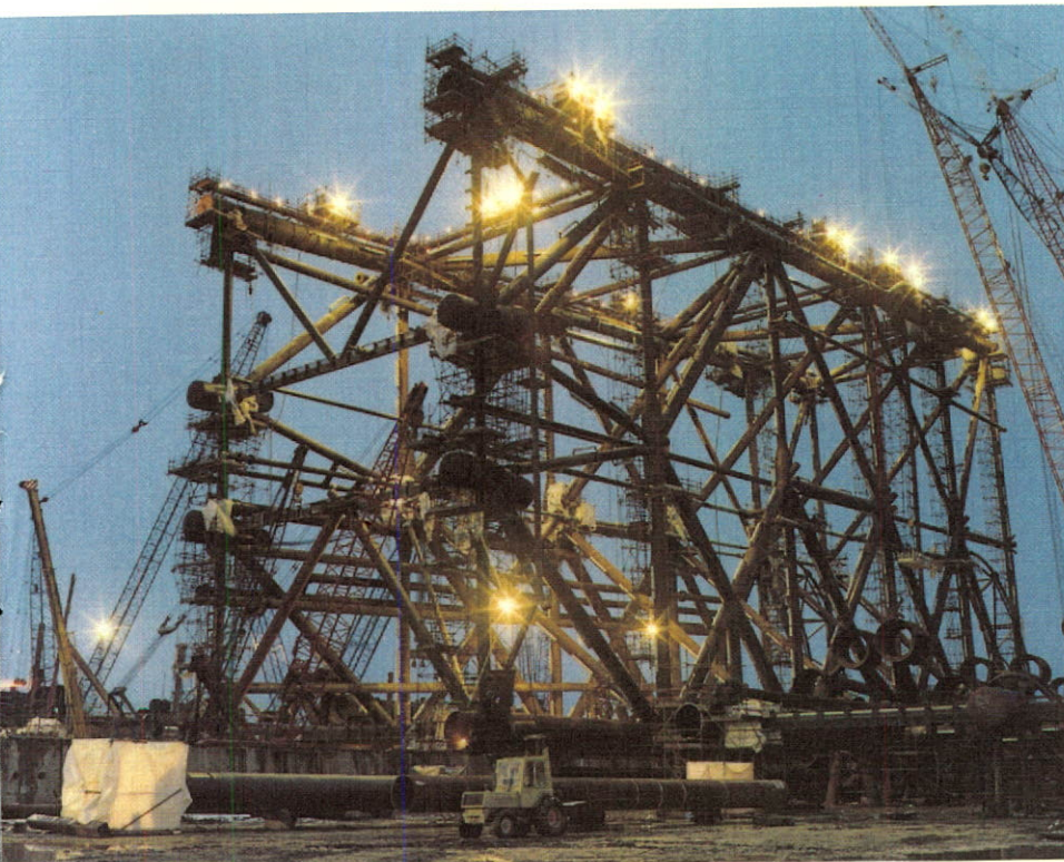
Steel jacket for self-contained drilling and production platform is shown under construction in Scotland. The barge-launched structure will be used in the North Sea's South Brae field.
