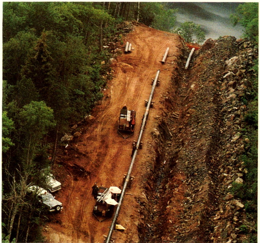
New construction in 1984 included work on this 330-kilometer lateral, built by Gaz Inter-Cité Québec, to provide natural gas to the Saguenay/Lac St. Jean region of Québec. The line was completely financed by a grant from the federal government. GICQ, in which ICG hold a 49% interest, delivered an estimated 800 million cubic meters (28 bcf) to more than 6,600 predominantly industrial customers during 1984.
