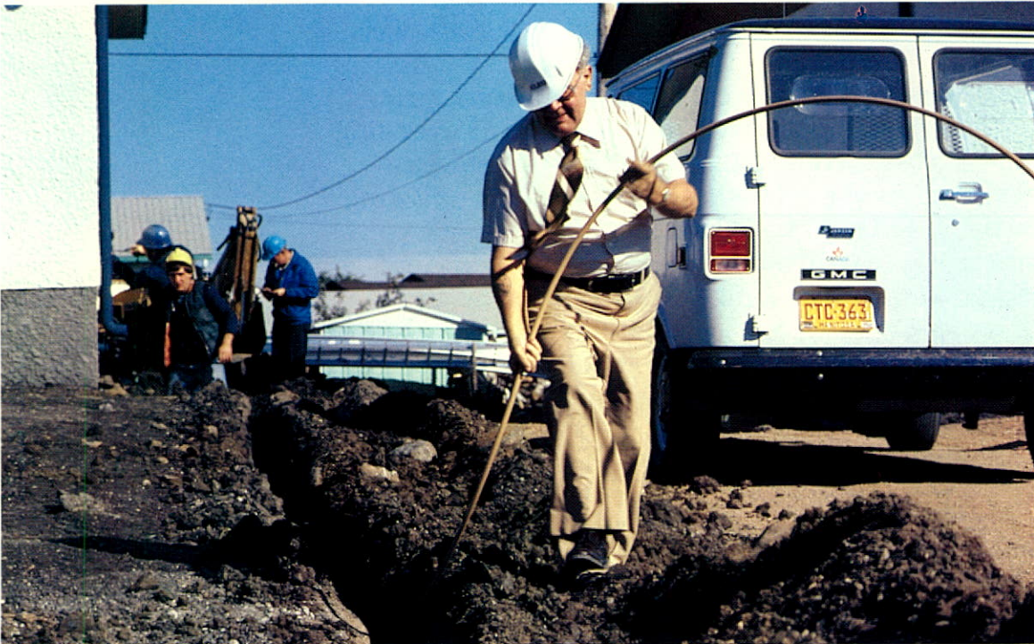
Natural gas service is being expanded to new customers in all ICG utility markets.
