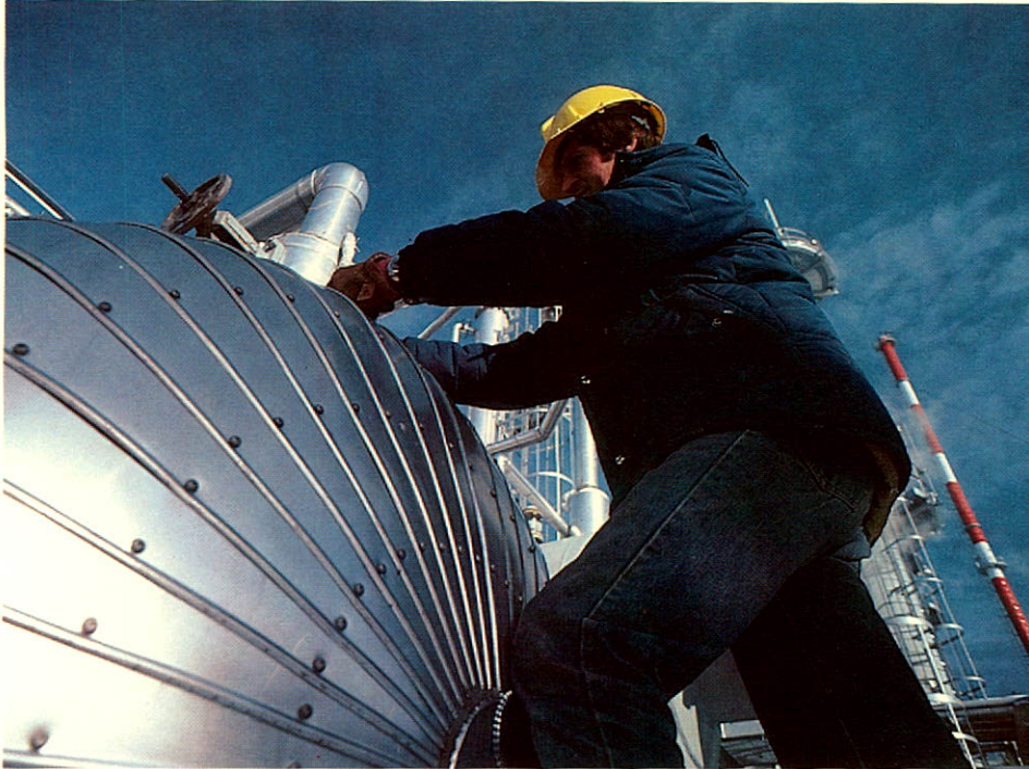
ICG has a 30% interest in the Rosevear gas plant which came on stream in 1980.
