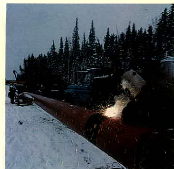
Side-boom tractors manoeuvre bent and weighted pipe prior to lowering. Backfilling is followed by cleanup and a rigorous site inspection program.
