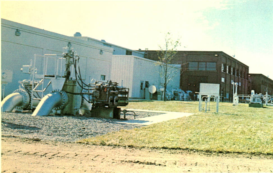
Deer River Pumping Station
