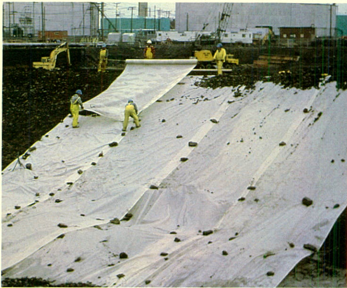
One of the geotextile fabric applications is for erosion control of river banks.
