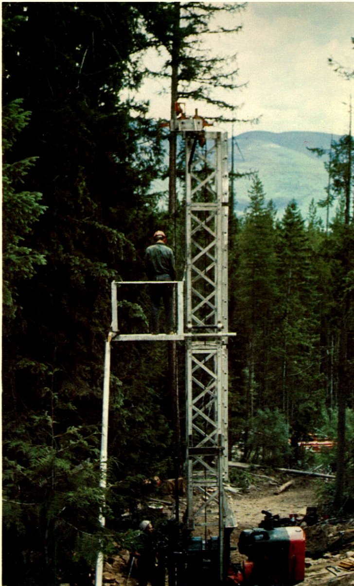
Connors Drilling Ltd. on a core hole contract in central British Columbia.
