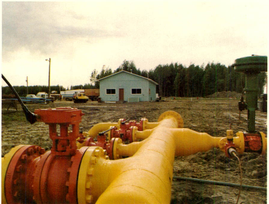
New gas gathering facilities at Wandering River in northeastern Alberta.
