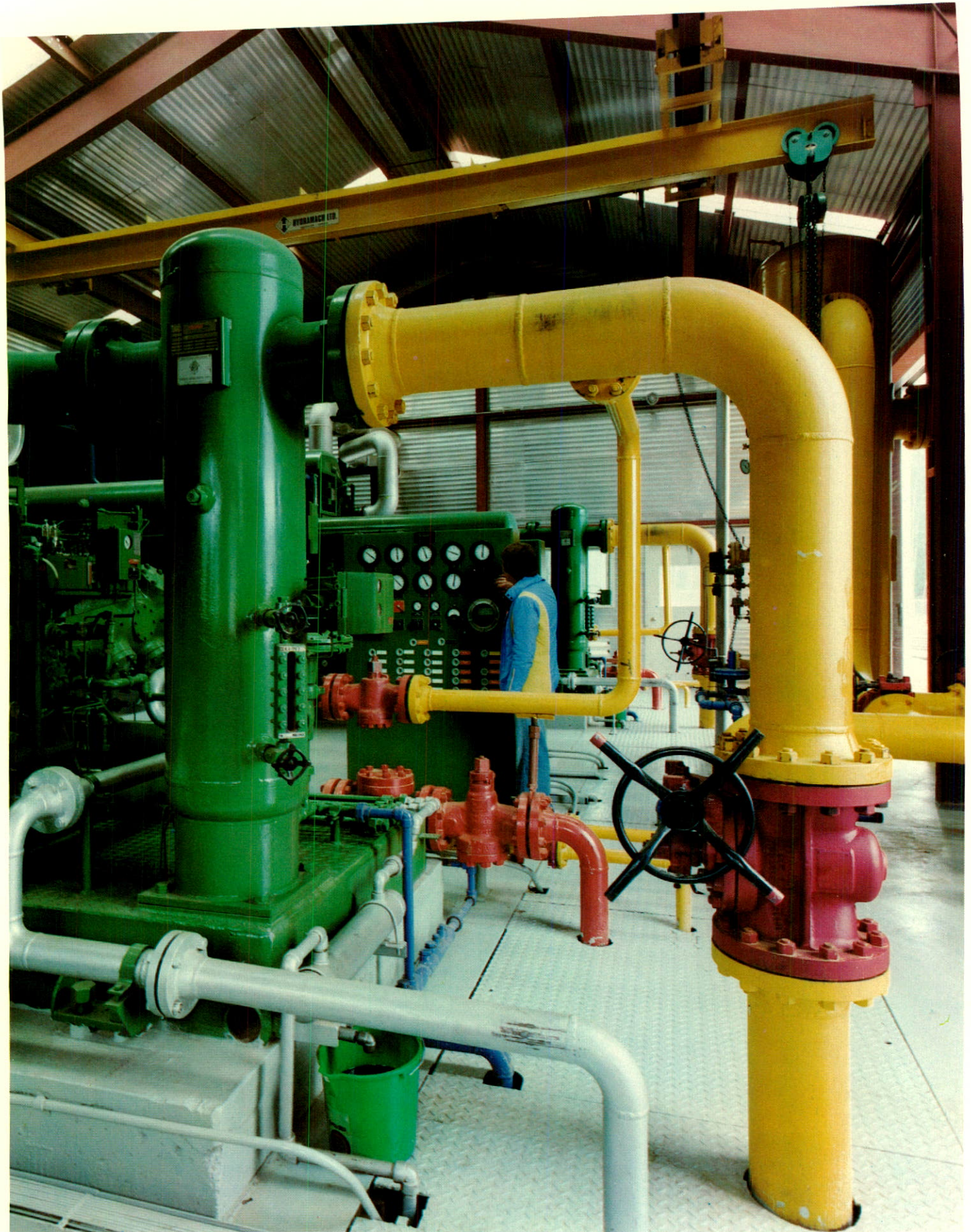
Wandering River gas compressor station. Bow Valley is the operator for a group of companies that own the Wandering River gas field, which is about 150 miles northeast of Edmonton, Alberta. The field commenced production in 1976 and is producing 22,000 Mcf per day to local markets. Gas is gathered from 37 wells connected to 64 miles of pipeline and collected at two central compressor stations; after processing and compressing to industry standards, the gas is sold to market.
