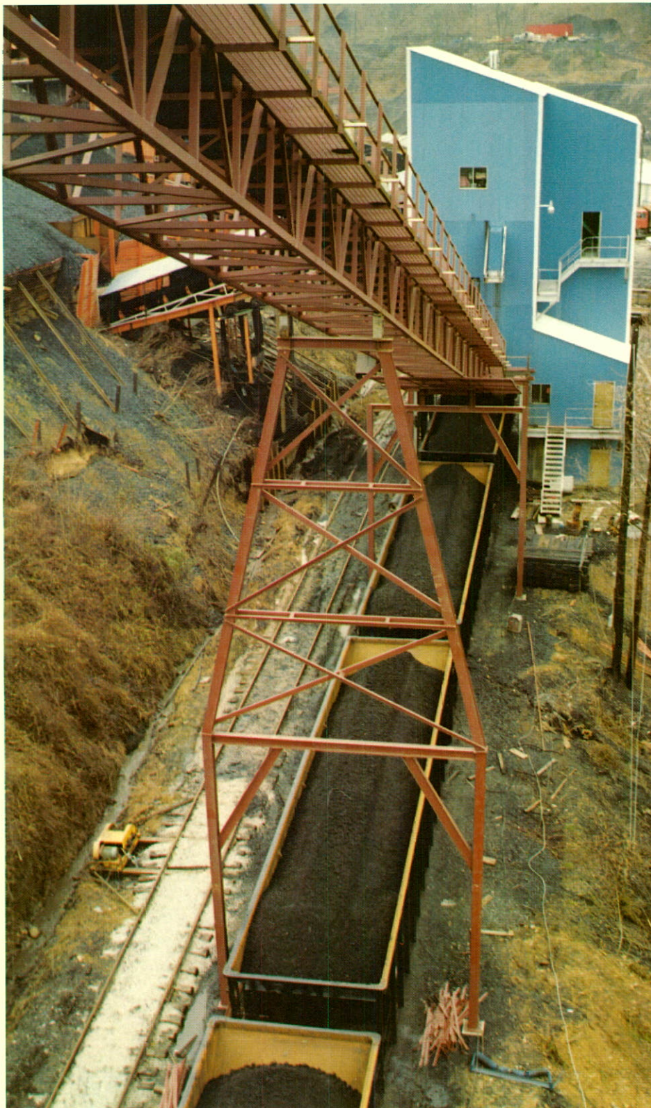
Bow Valley's new automatic weigh bin and coal loading facility in Harlan County, Kentucky.
