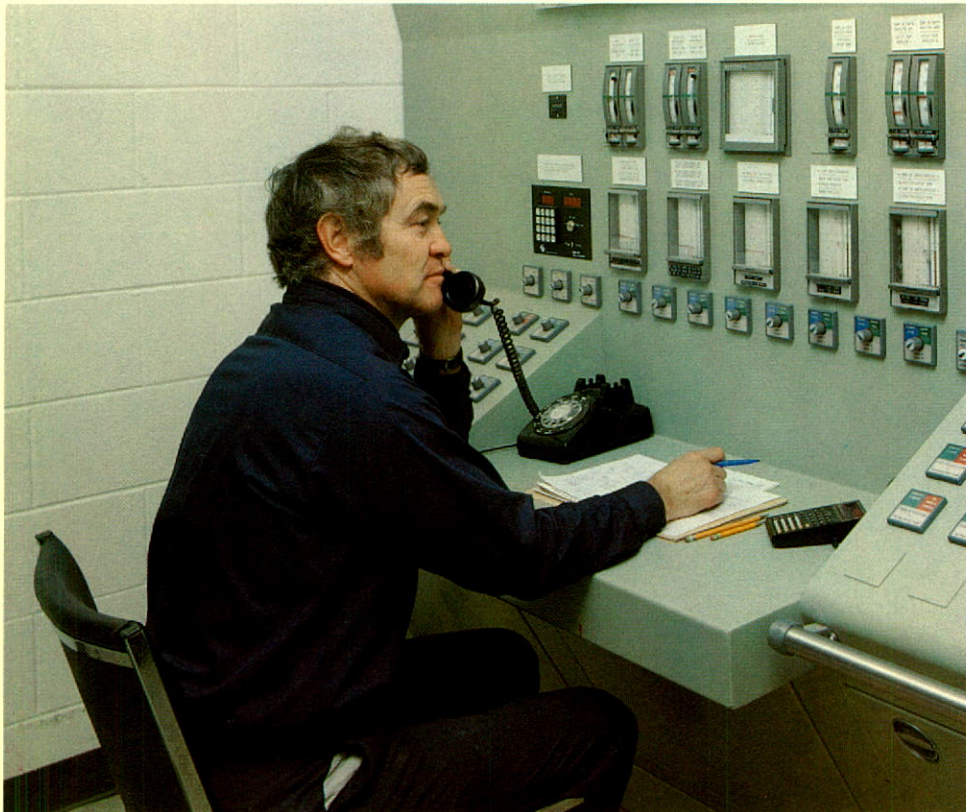
The control panel of Montreal Refinery's effluent upgrading unit, which was commissioned in 1979. This BP-designed plant features sand filters, and "biofilters" in which bacteria are grown to remove contaminants from the water before returning it to the St. Lawrence River.
