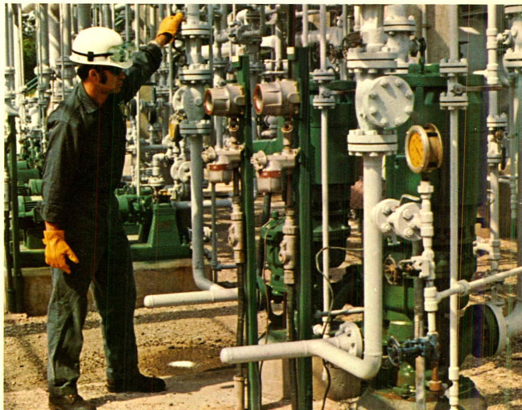
This plant, commissioned in 1971 at Trafalgar Refinery, produces chemical-grade propylene. The propylene is sold in the United States to The Standard Oil Company (Sohio), an associate of The British Petroleum Company Limited, which uses it to manufacture acrylonitrile, an important raw material for the synthetic rubber and textile industries.
