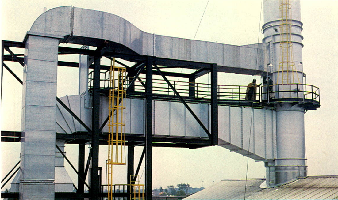
This air preheater, which conserves energy and improves the efficiency of a crude distillation unit at BP's Montreal refinery, was commissioned in October.
