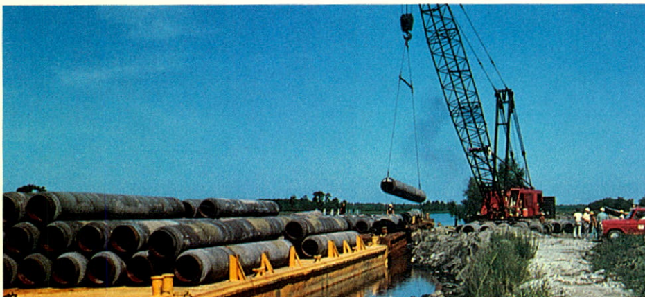
Concrete pipe is loaded aboard barges by an Anchor Wate crane at Belle Chasse, Louisiana. Anchor Wate is part of Canfarge's Permanent Concrete Division.
