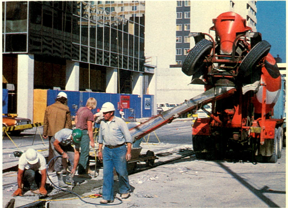
A Conmac truck delivers concrete to a project site in Calgary, Alberta. Conmac is a division of Canfarge, a subsidiary of Canada Cement Lafarge.
