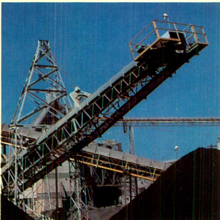
The coal unloading system at the Forth Worth Plant, Texas.
