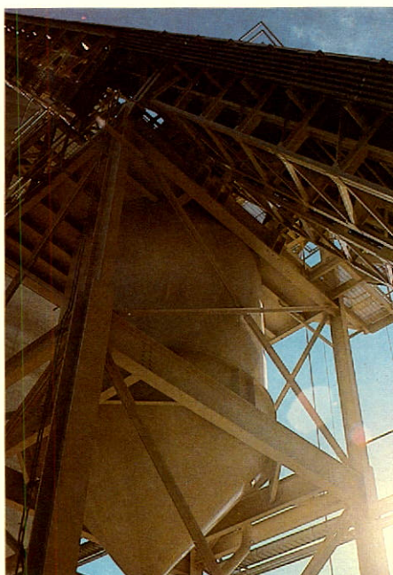
A loading hopper at the Balcones Plant, Texas.
