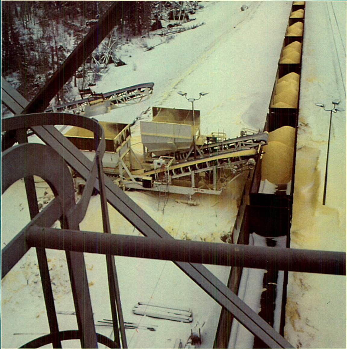
Temporary facilities being used to load sulphur onto a unit train at Ram River while new facilities are under construction.
