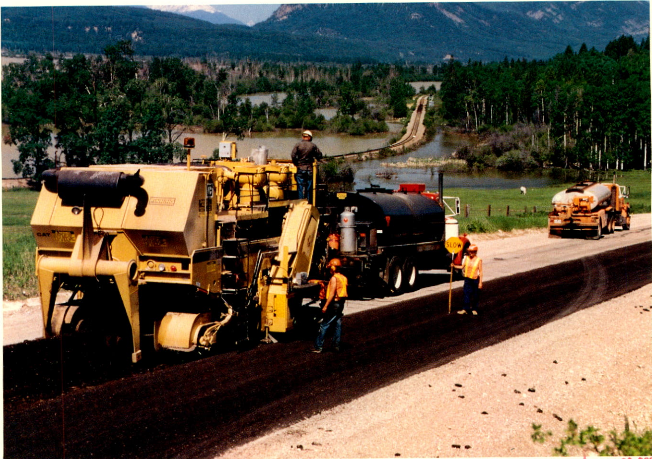
New technique in resurfacing highways was tested. Work was done with a big spread of Caterpillar paving equipment.
