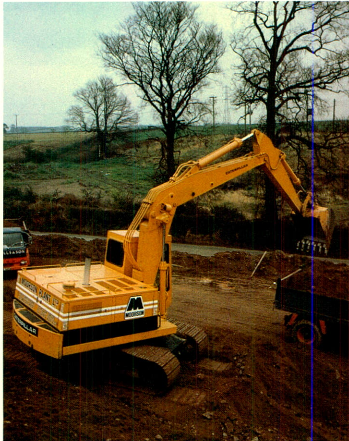
Caterpillar 215 hydraulic excavator moves material for reinforcement of roadbed eroded by flood waters.
