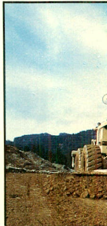
Caterpillar motor grader helps maintain haul road at Revelstoke Dam site scheduled for completion in 1985.
