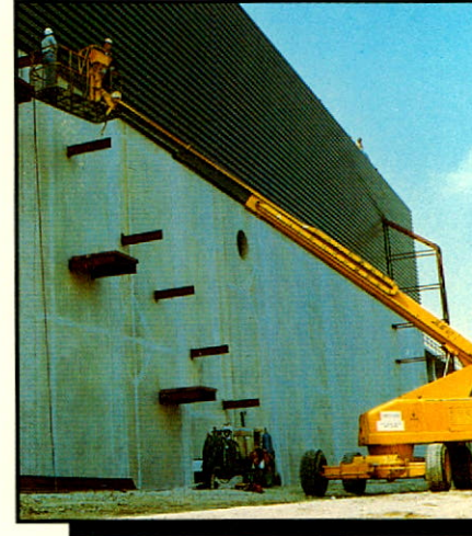
Sixty-foot reach of JLG high lift equipment allows welders easy access to outside stairway installation at new food distribution plant.
