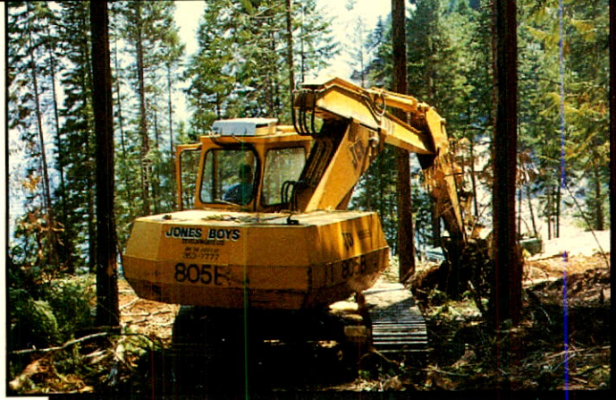
JCB 805B hydraulic excavator clears land for residential subdivision above Kootenay Lake.
