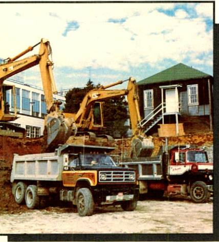
Twin Caterpillar 225 excavators work side by side in building project at the University of B.C.
