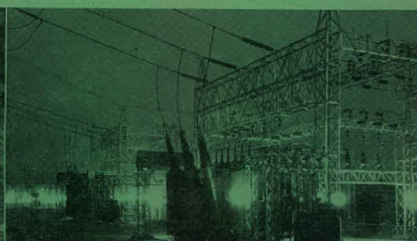
The new Horne-Payne, largest outdoor substation in the Canadian West
