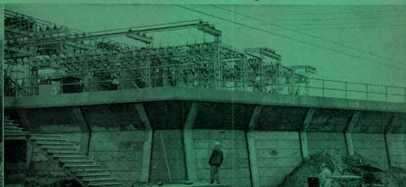
Sperling Substation, another new link in Greater Vancouver's sub-transmission "ring"
