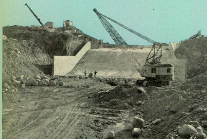
THE SPILLWAY SECTION of the Wahleach Dam under construction. This clay-core, rock-filled structure, 1,375 ft. long and 55 ft. high will raise the lake level 40 ft.
