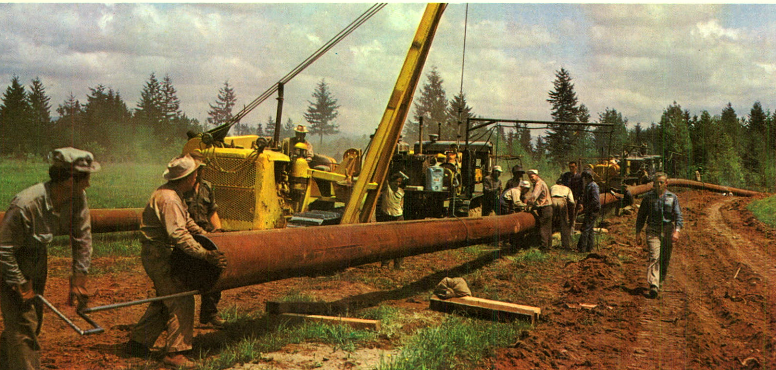
The trunk pipeline carries natural gas 36 miles from Huntingdon, near the United States border, to the "city gate" on the south bank of the Fraser River near New Westminster.
