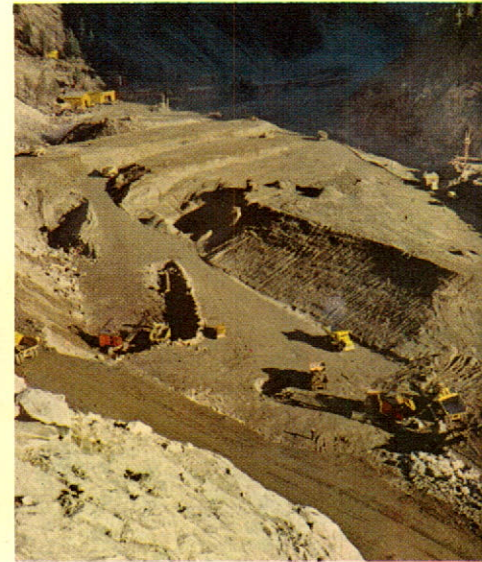
At Bridge River, this new dam will store an increased head of water to drive turbines in a second power station, now under construction, and raise the capacity of the existing plant.
