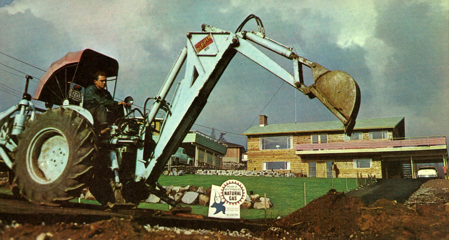
598 miles of mains were laid in 1957 to bring the benefits of natural gas to more customers.
