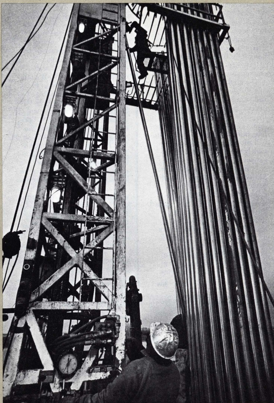
Near Kindersley, Saskatchewan, drill rig crew prepares to drill another well for Westar Petroleum, a wholly-owned subsidiary of B.C. Resources, which operates about 400 oil wells in the region.
