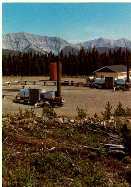
This gas facility in the foothills of southern Alberta is one of several operated by the Company.
