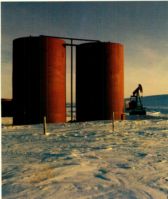
Production facilities at Wood River, Alberta.
