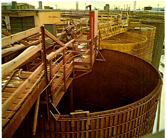
100,000 gallon storage tank at Northern Pigment
