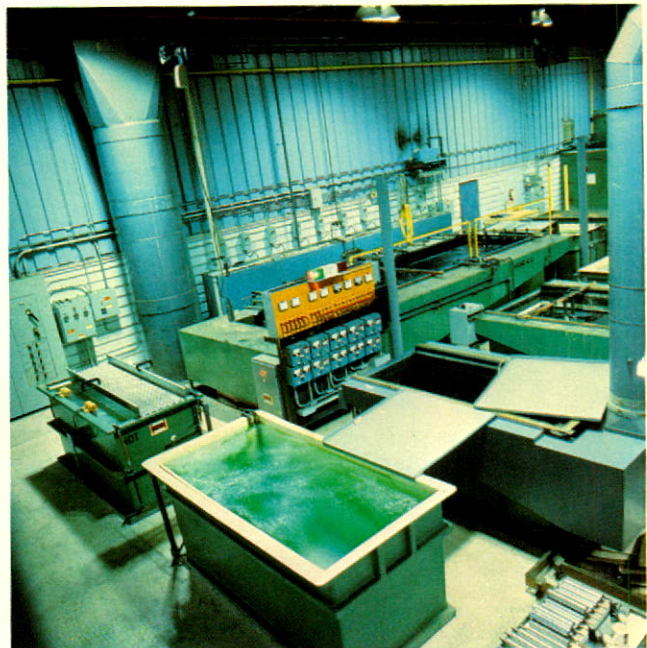
New installation at Neo's Saltfleet plant for plating aircraft landing gear components.
