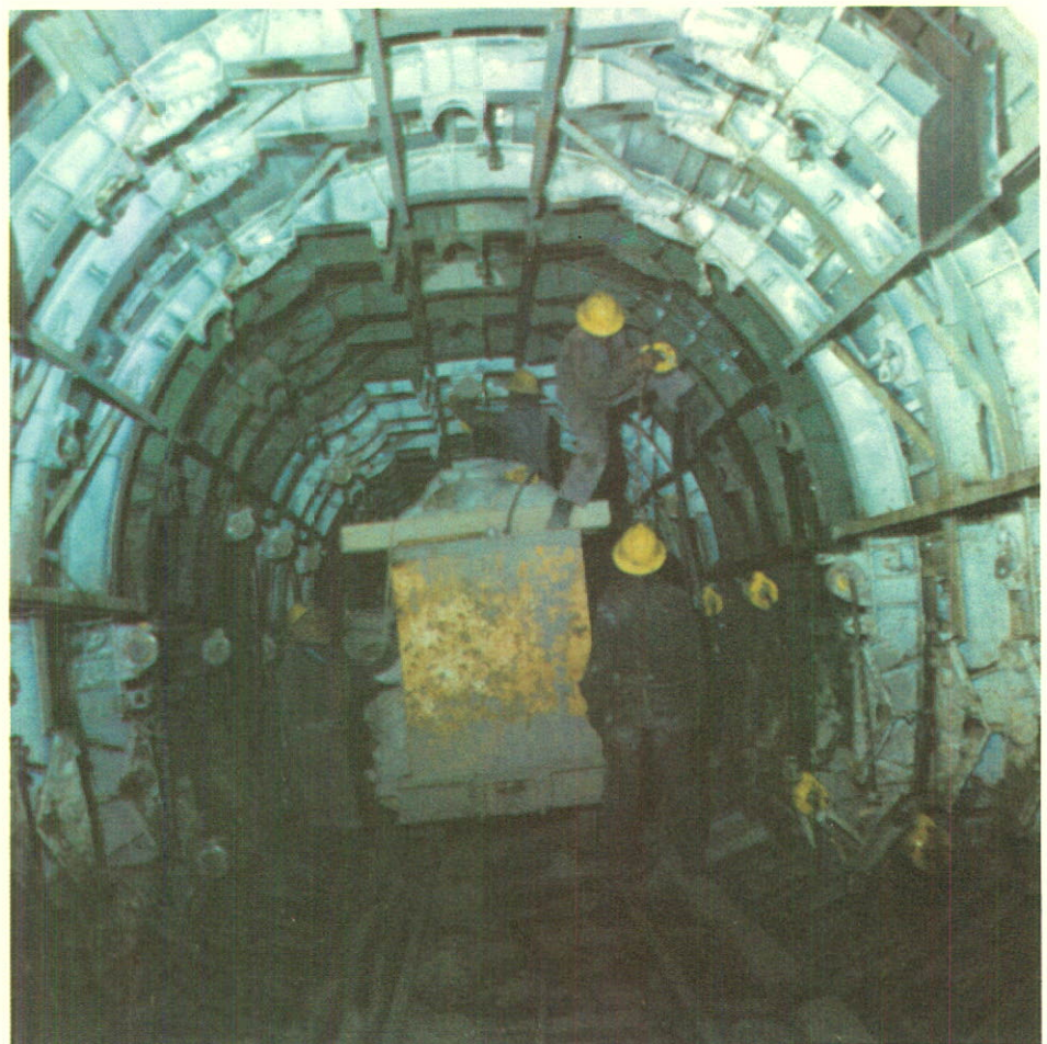
Construction scenes of the Majes irrigation project in Peru involving the services of Foundation Company of Canada Limited.
