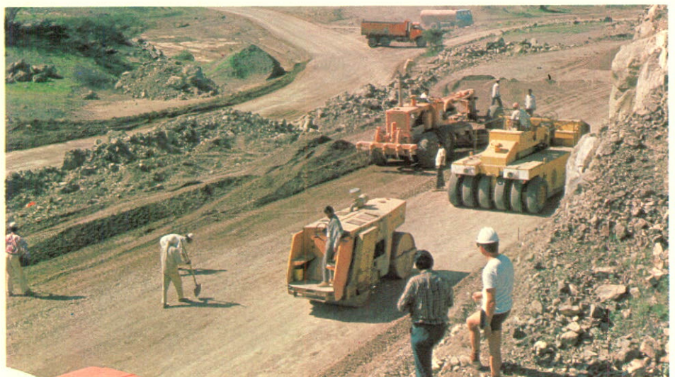
Road Construction in Oman involving the services of Cansult Limited of Toronto.
