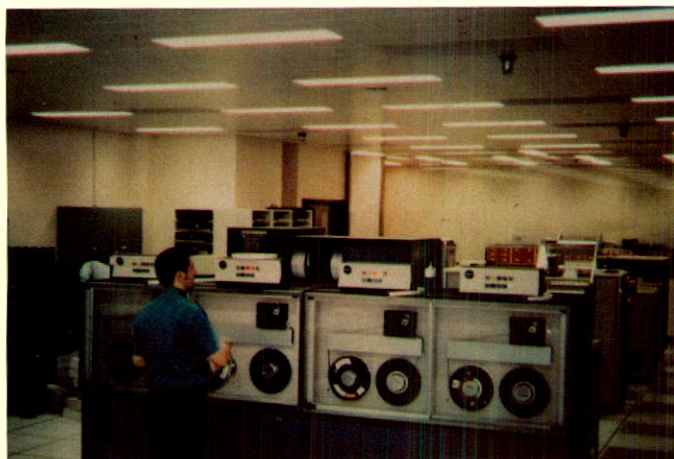
The Co-operators Data Centre
