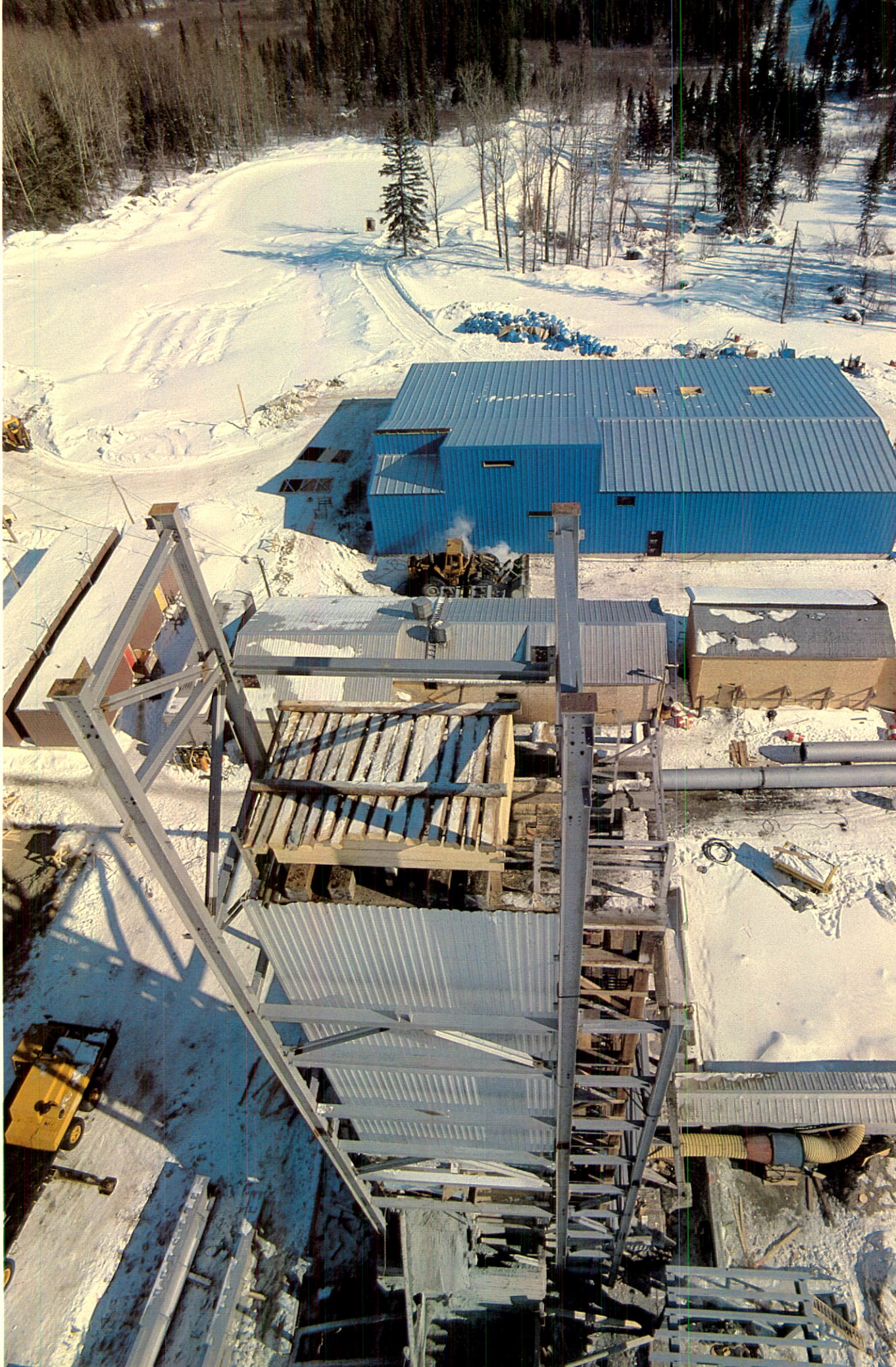
Construction at the Holt-McDermott Mine with new hoist room in the background.
