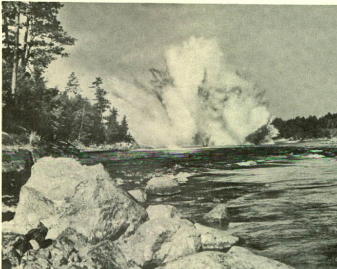
Underwater blasting of rock, Winnipeg River near Kenora, Ontario, to provide ditches in which to lay dual pipe.
