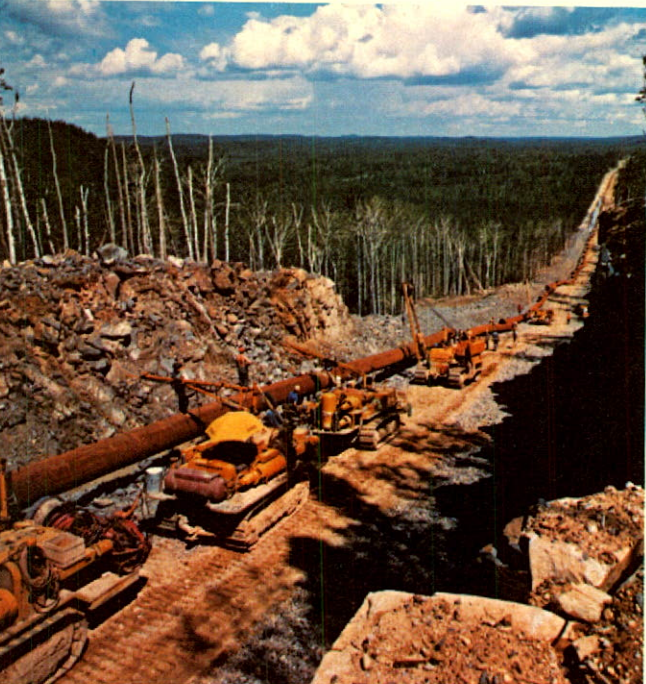
From left to right: 24 inch diameter pipe being laid on a hill during looping near Trenton, Ont.; ditching machine at work in Saskatchewan; bottom: welders at work through the rock country of northern Ontario.
