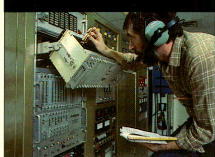
Top: Testing new graphic control panel. Station 21, Grenfell, Saskatchewan.
