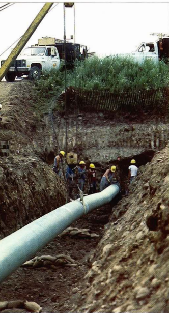
A work crew replaces a section of pipe at a road crossing near Cobourg, Ontario.
