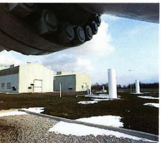
Compressor station 13 at Otisville, Michigan, is one of 14 on Great Lakes Gas Transmission Company's pipeline which stretches from Emerson, Manitoba, to Sault Ste. Marie and Sarnia, Ontario, via three Midwestern states.
