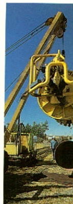
The ends of the pipe are cleaned and bevelled for a snug, secure fit.
