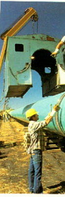
The pipe is joined together by automatic welders housed in special huts lowered over the pipe.
