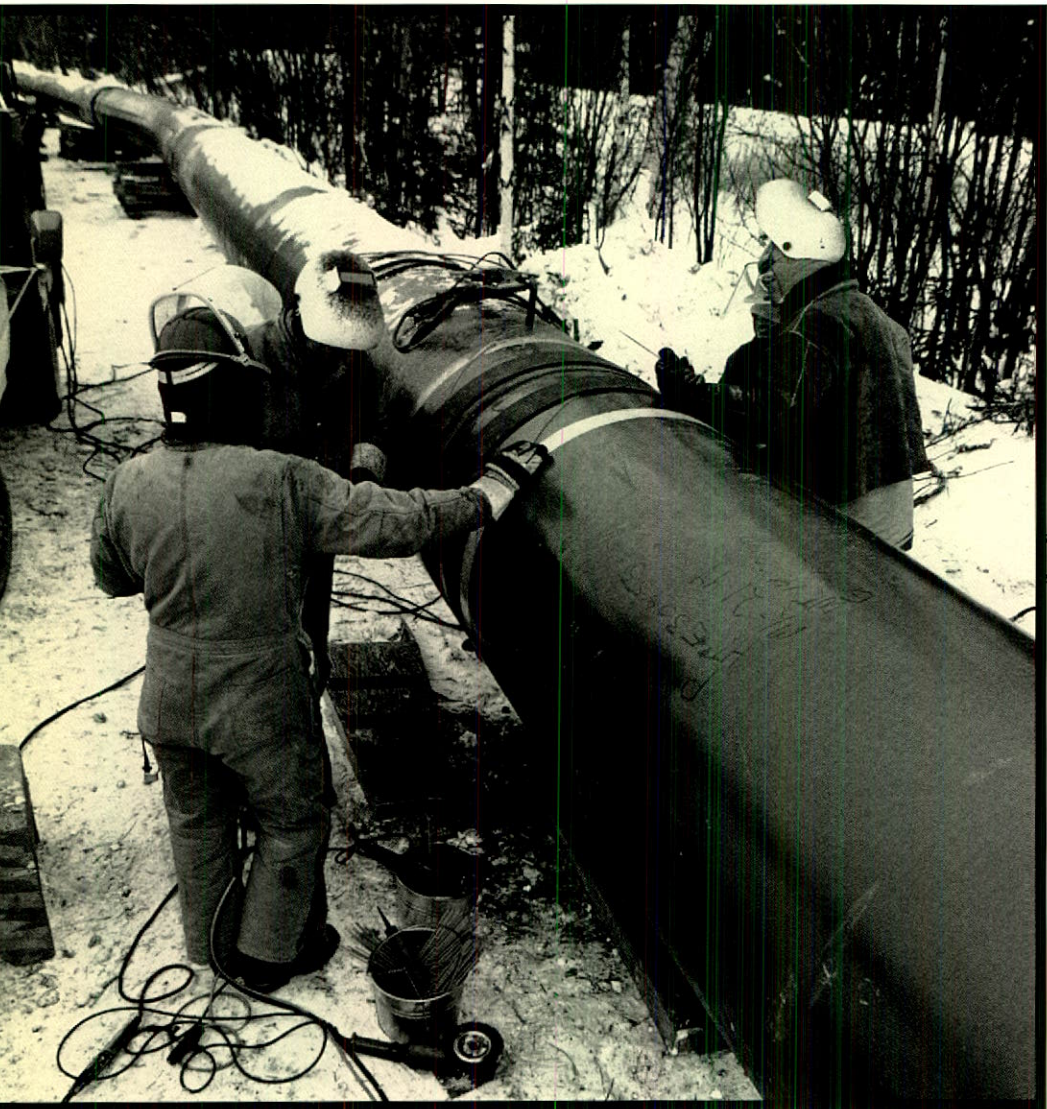
In 1993, TransCanada installed 580 kilometres of pipe in four provinces across terrains ranging from the Prairies to the Canadian Shield.
