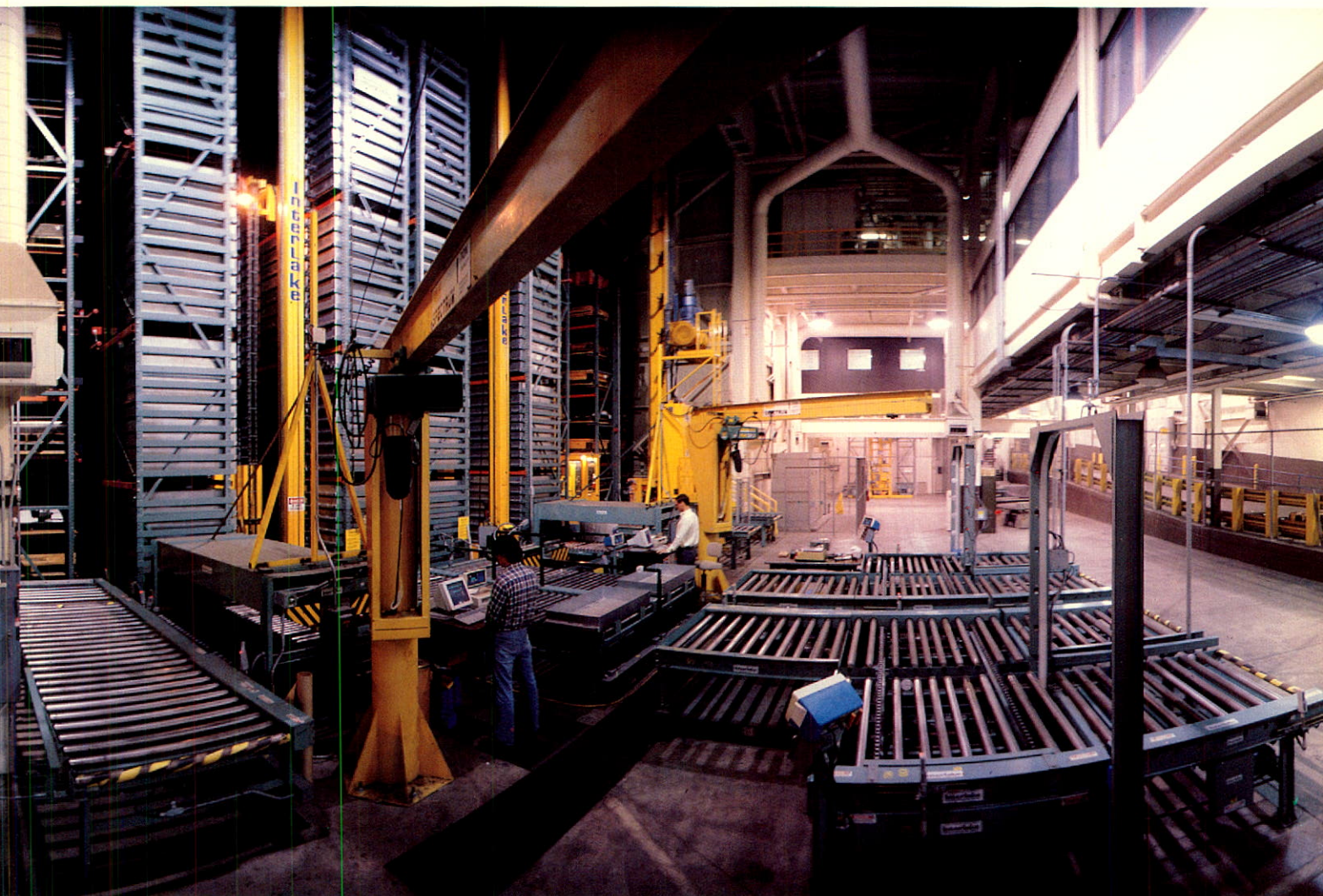
A 210-degree panorama at the U.S. Army's Rock Island Arsenal is filled with Interlake Material Handling products integrated into a system including conveyors, automated storage and retrieval, automated guided vehicles and rack.
