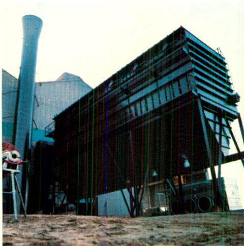
At Riverton, N.J.—the new modern system for air and water pollution control.
