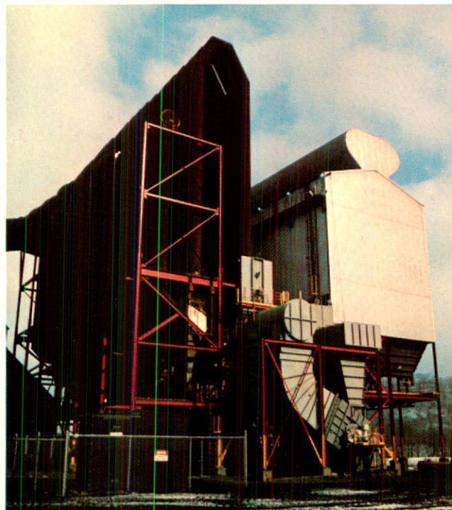
At Beverly, Ohio— a $2.6 million environmental control installation.
