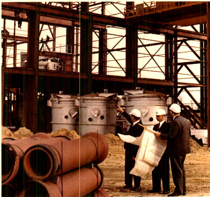
Construction is nearing completion on this new $8 million plant at Riverton, N.J., where atomized powders will be produced.
