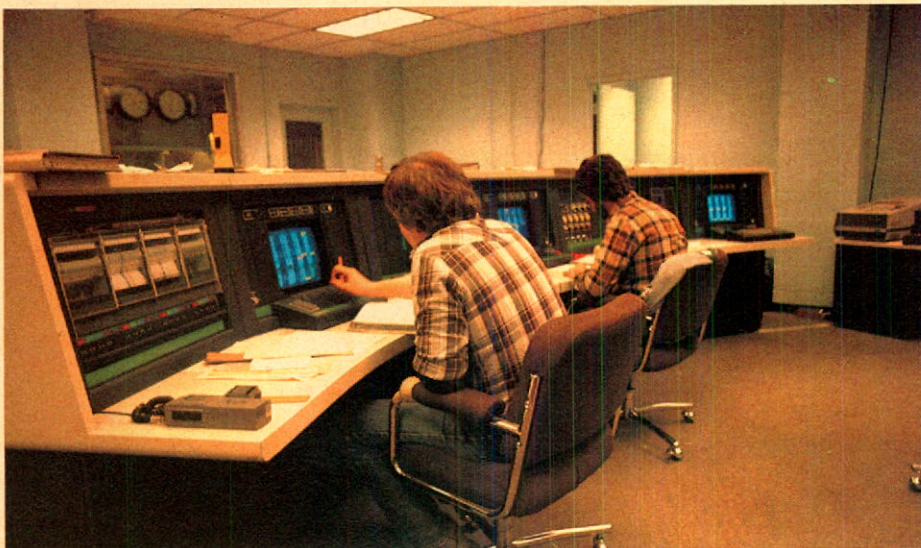
Modern control room panels keep operators informed on process changes and problems reducing reaction time to implement changes.
