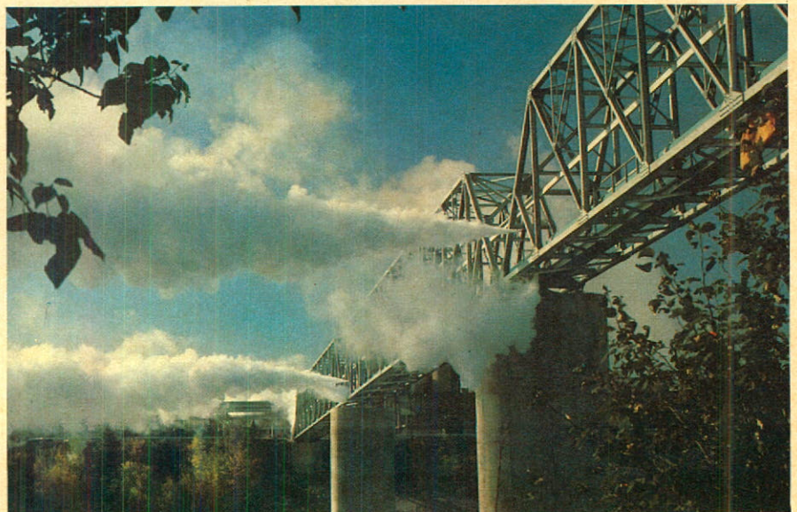
Steam pipeline being cleaned by blowing out at pressure prior to coming online
