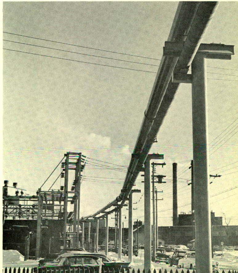
Chips from the Hardwood Woodroom at Cornwall are blown through this 18 inch pipe for a distance of 1,800 feet.
