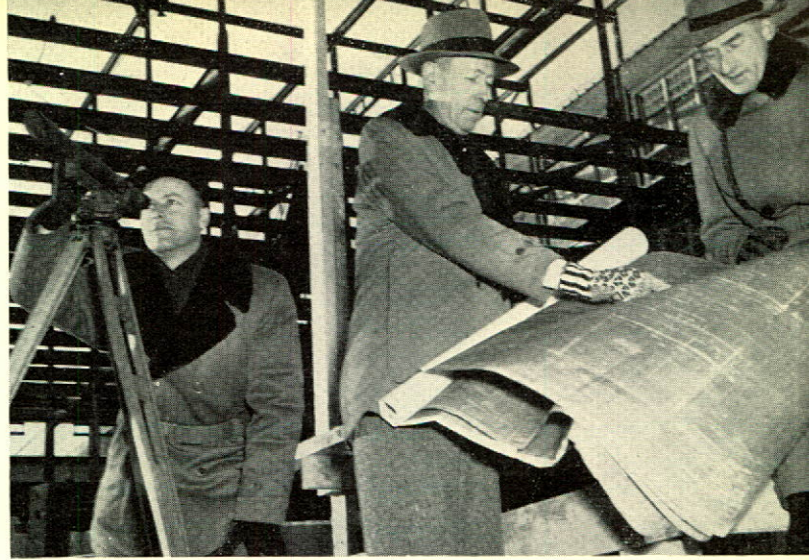
Addition to the Stock Preparation Room under construction at the Cornwall Division. Engineer J. E. Pescod adjusts his level, while Chief Draughtsman R. W. Boland and Field Engineer H. De Wolfe examine the blueprints.
