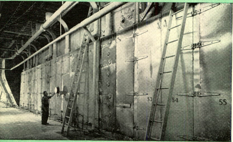
The tunnel dryer which extracts the moisture from the wet Insulating Board.
