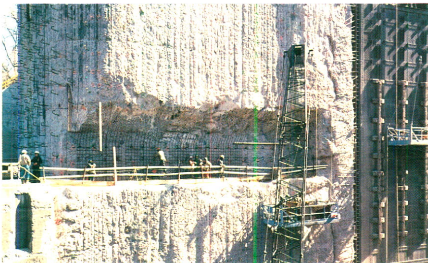
Welland Canal rehabilitation: Workers install steel reinforcement to lock wall prior to refacing.
