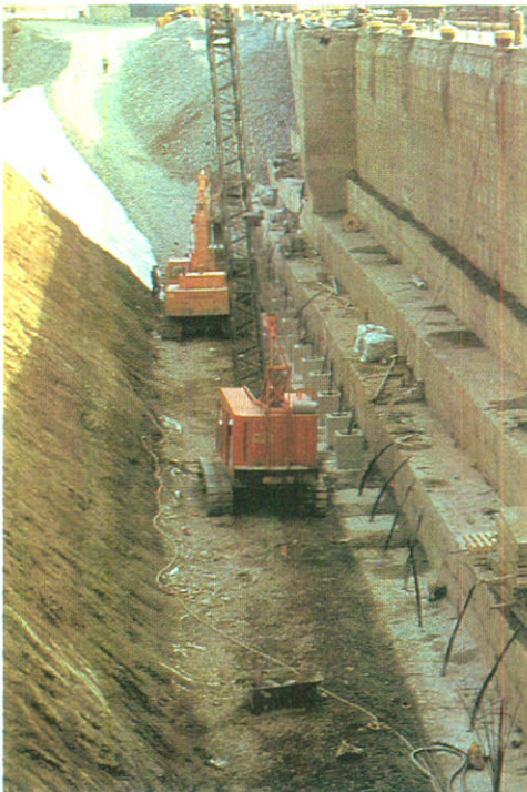
The Welland Canal Rehabilitation Program calls for the uncovering of the back face of lock walls prior to the installation of reinforcing rods and ground water drainage systems.
